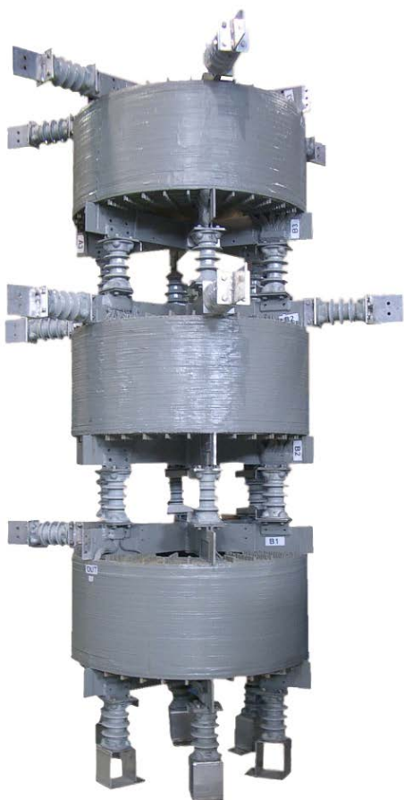
Figure 1: 3 phase outdoor current limiting reactor
